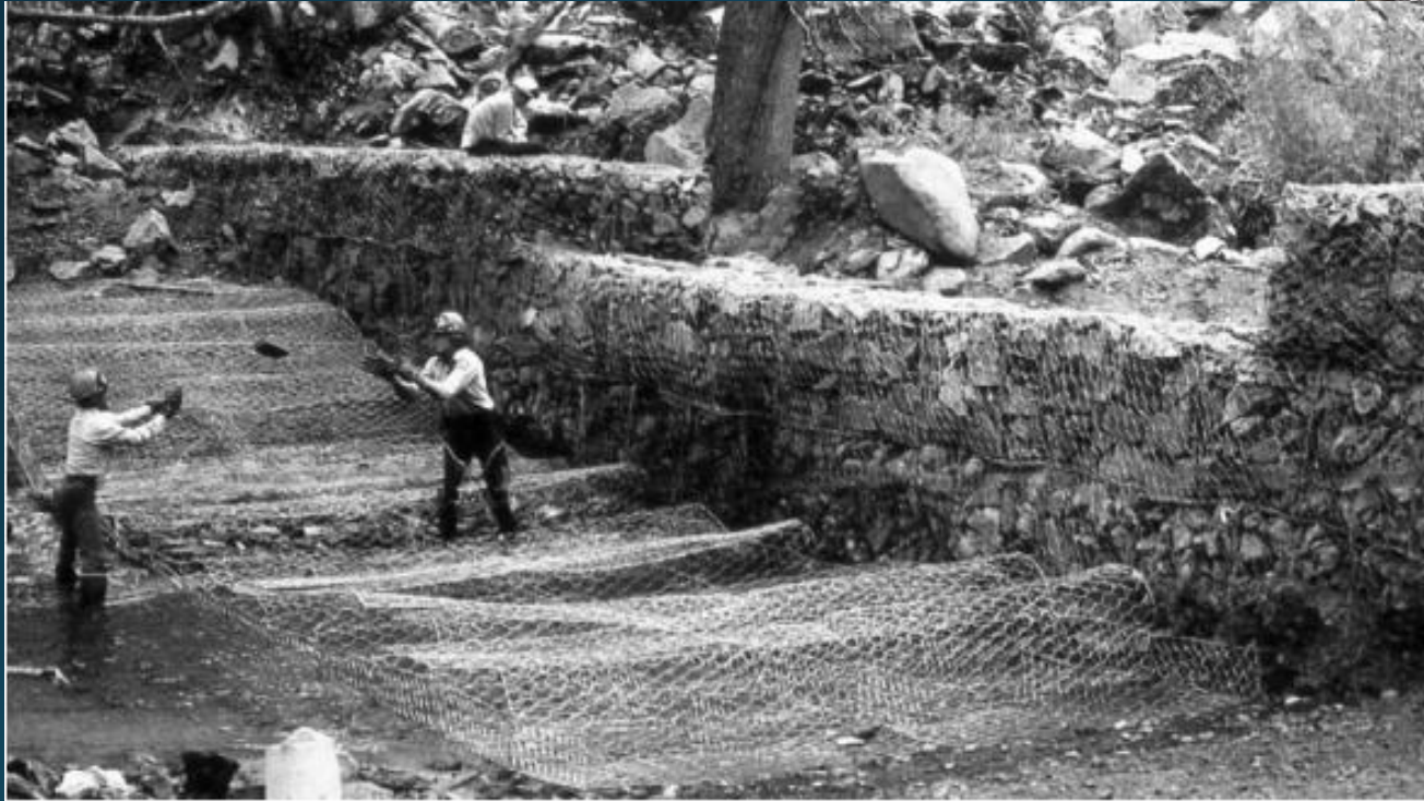
12 - Schaeffer Barrier showing gabion basket construction completed 1983. September 1983. Photo courtesy of INF.
